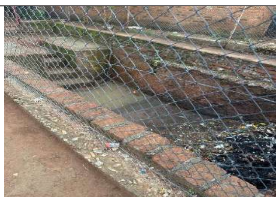
Poor Waste Management at Buyinja HCIV
