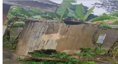
Bubulo HCIV: Dilapidated water tank for demolition
