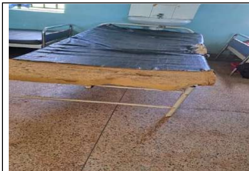
Dilapidated beds and torn mattresses in Wakiso HCIV maternity ward
