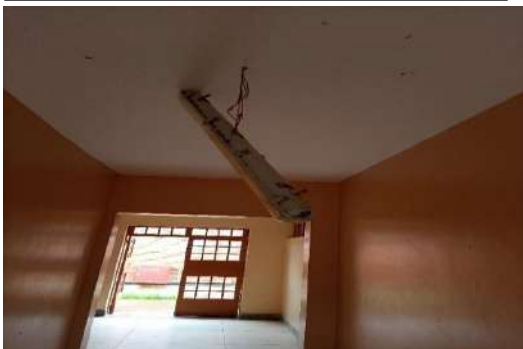
Loose/falling electrical fittings at Isolation center-Entebbe RRH
