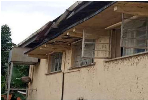
A dilapidated office block at Grade A -
