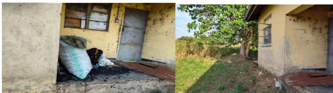
Angangura HCIII- dilapidated staff accommodation
