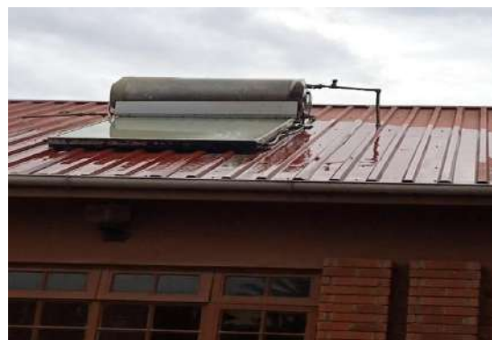
Leaking water pipe of a solar heater at Isolation Center-Entebbe RRH
