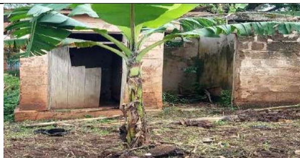
Non-functional pit latrine at Busawamanze HCII
