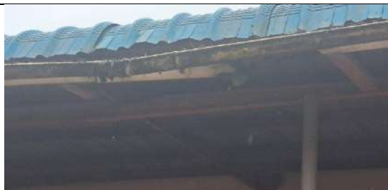
Sulking gutters in Wakiso HCIV.
