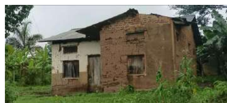
Bubulo HCIV: Dilapidated staff house for Demolition
