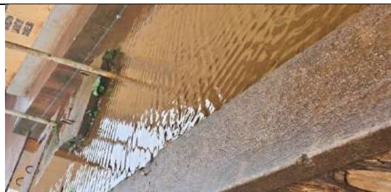
Water logged Veranda of the OPD Wakiso HCIV
