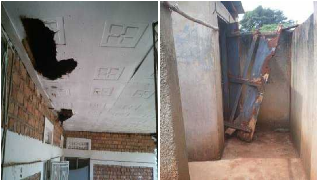
Ceiling damaged by bats in Kiziko & latrine door damaged by termites in Butaka
